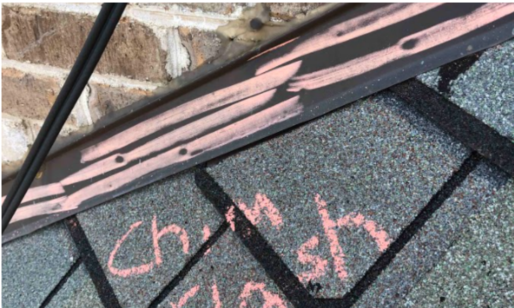
Fig 2. Chalking metal surfaces reveals dents in metal chimney flashing
