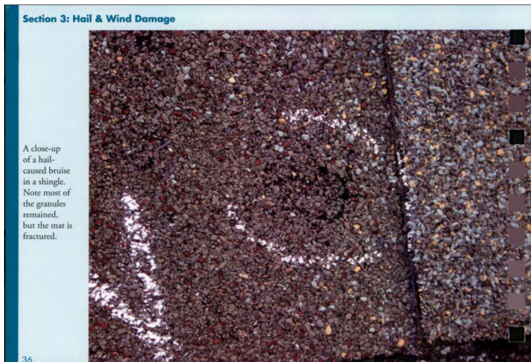
Fig. 1: Circular to semi-circular impressions in shingle surfaces indicate hail damage.
